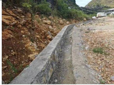
场内截排水沟
